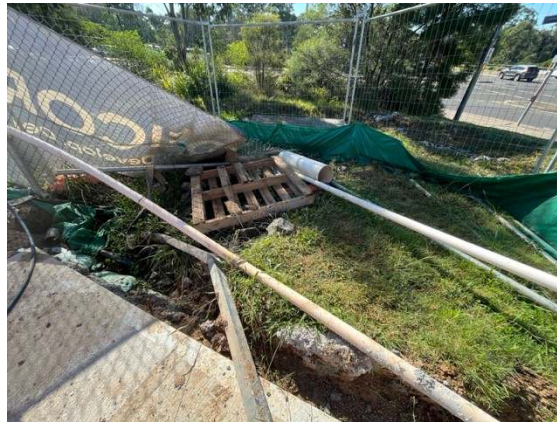
Photo 19: Site 2 – Clean-up of discharge point required including replenishment of ballast, removal of redundant pipes and re-establishment of boundary and sediment fencing
