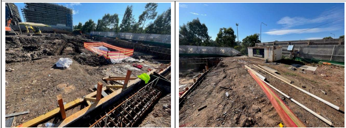
Photo 17: Sediment basin set-up in basement excavation for Stage 2B, 2C, 2E. Improvements to sediment basin formation required to comply with the
